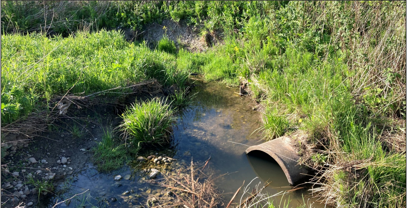
Photo 3: The iron pipe railway culvert at the head of the watercourse segment at the site and its little scour pool. The downstream channel is in the photo background, perpendicular to the culvert orientation.
